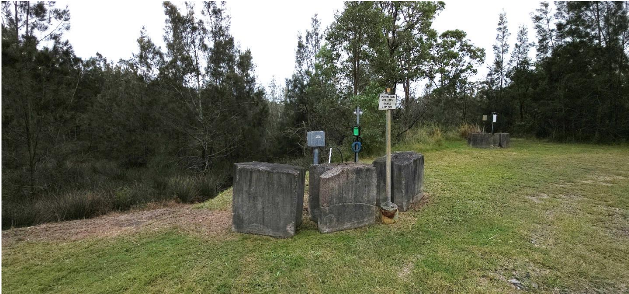
Plate 3 Water flow meter at LDP of EPL 9
